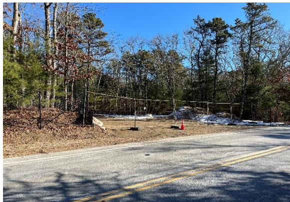
944 Shootflying Hill Road Pump Station
